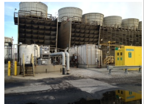
Marley Tower chemical feed
