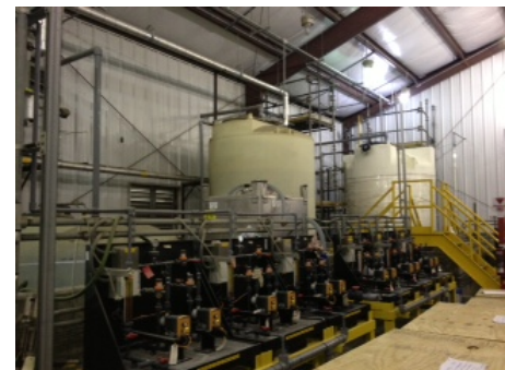
Chemical tanks and pumps
