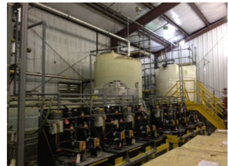
Chemical feed tanks and pumps
