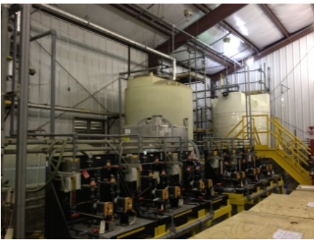
Chemical tanks and pumps
